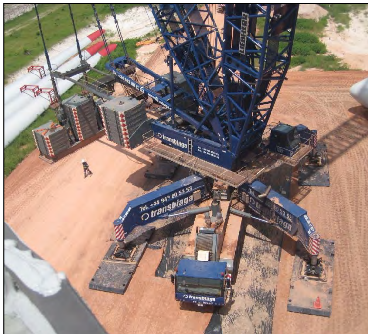
Fig. 26 Example of a crane installed on a platform.
